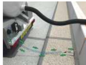
Continuous Ground Loop Monitoring check
